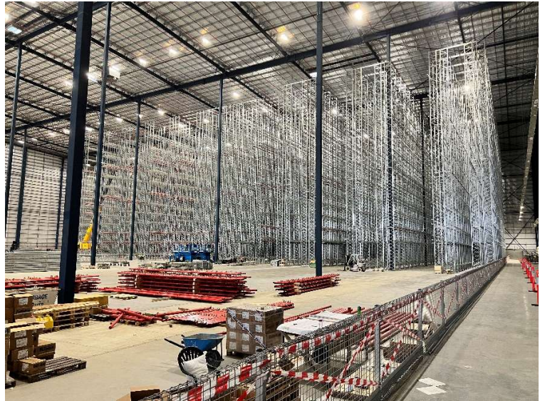
High Bay ASRS Pallet Racking for Bito Lagertechnik
